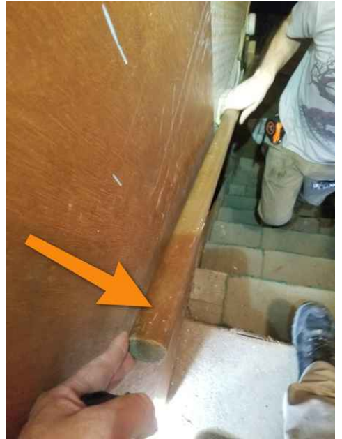
Basement handrail is extremely flexible and is only fastened in the center. It does not provide adequate support.
